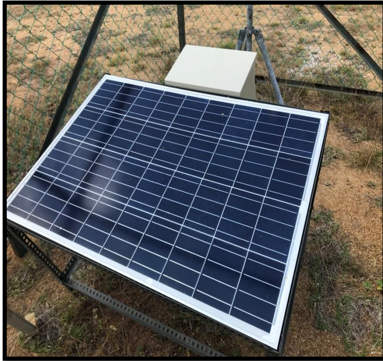
Figure 4.13: Solar panel that is installed to link with the weather console
