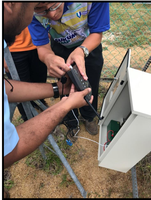
Figure 4.12: Linking the weather station console to the solar panel
