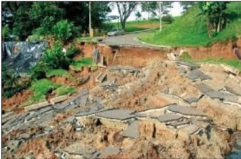
Figure 2.4: The erosion caused by shear strength fail.
