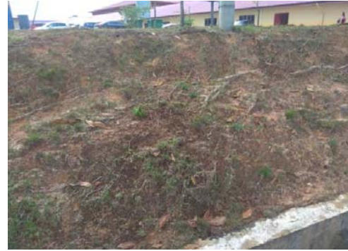
Figure 1.2: Shows the roots of the vegetation exposed
