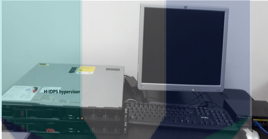
Figure 4.3 Two HP servers.
