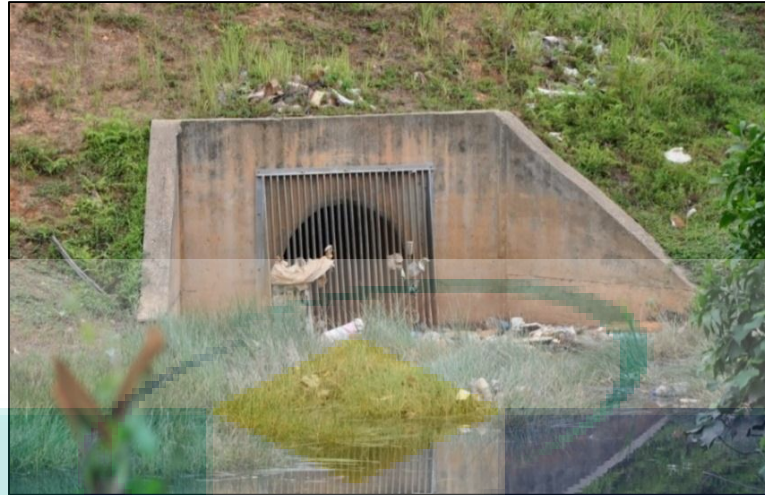
Figure 4.43 The culvert discharging to the stream is provided with steel screen to trap rubbish at the side of KM 5 Gambang-Kuantan, Kuantan, Pahang
