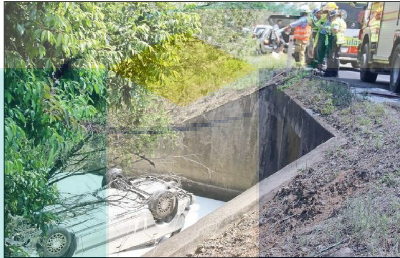
Figure 4.41 A car plunged into culvert opening at South of Gympie, Queensland, Australia on 17 November 2012
