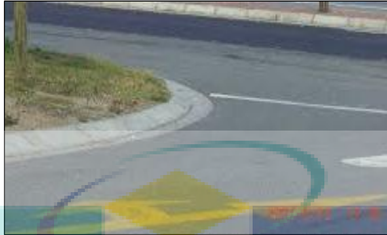
Figure 4.50 Kerb is more forgiving with low drop level, tapered with the provision of slight depression for drainage at Port Elizabeth, South Africa
