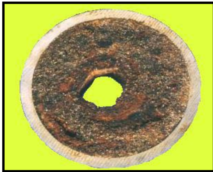
Figure 2.3 Wax Deposition (Phillips Petroleum Co.)
