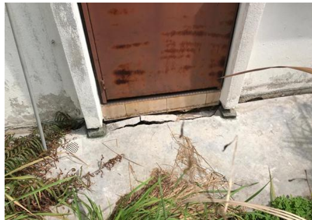
Figure 12. Splitting between ground floor and wall
