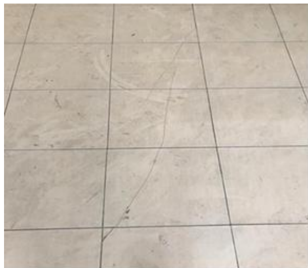
Figure 13. Cracking on the tile and floor
