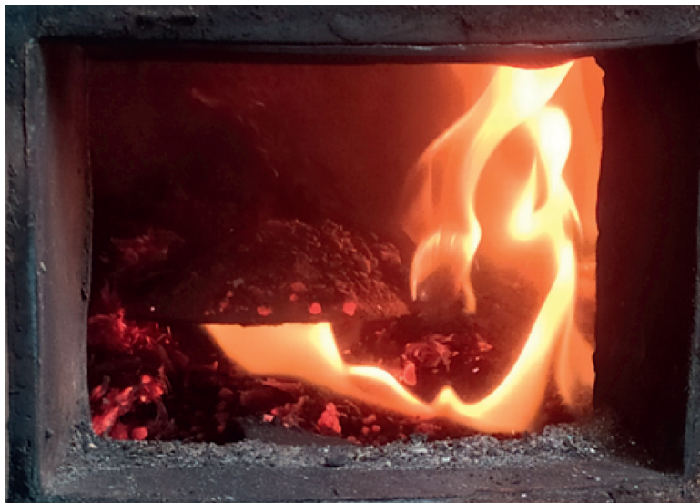
FIGURE 15: Display of combustion fire in the combustion chamber.
