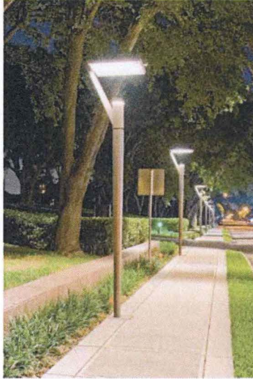
Figure 2.1 LED lightings installed along the Houston Uptown district sidewalks.
