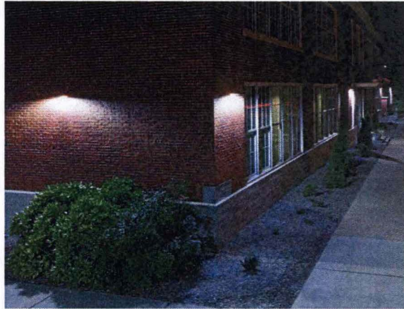
Figure 2.5 Wall-mounted lighting application on the exterior wall of the building. Source: Stouch Lighting (n.d.). Wall Pack and Building Lights Definition.
