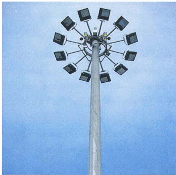
Figure 2.4 High mast light poles used for illuminating over large area. Source: Valmont Industries, Inc. (2018). Lighting: High Mast Lighting.
