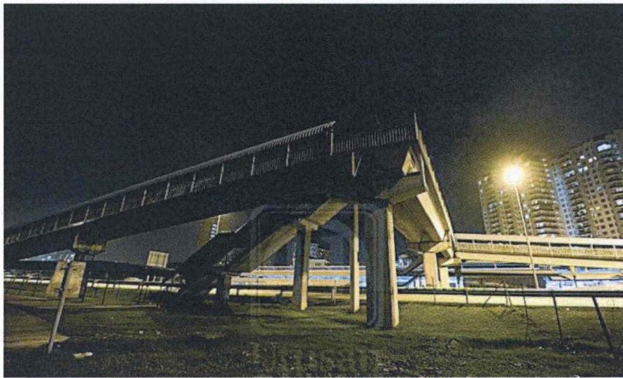
Figure 2.6 The pedestrian bridge in Kuala Lumpur which is not well-maintained and poorly-lit
