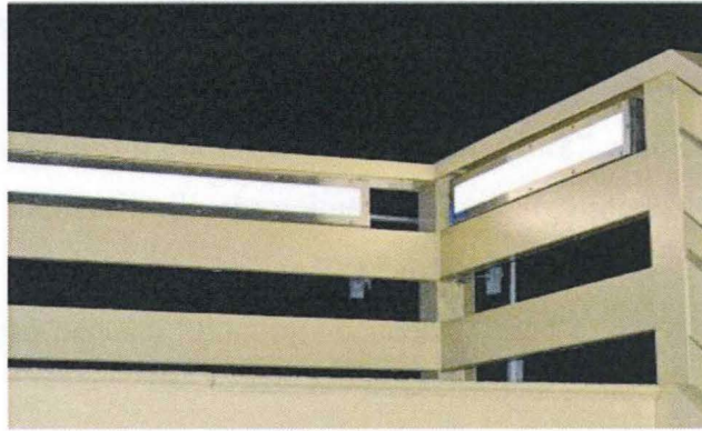
Figure 2.9 A close up on the J9 Series luminaires installed along the pedestrian walkway of Market Street Bridge.
