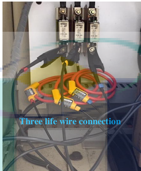
Figure 3.13 Fluke 437-II Power Harmonic Analyzer cable setup for three-phase connections.
