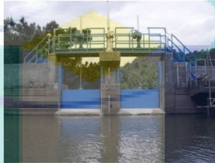
Figure 2.4 FRP water gate at Komagari dam Source: Nishizaki (2009).
