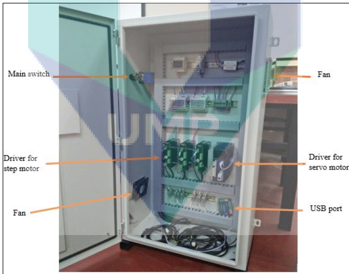
Fig. 28 Control Panel Box
