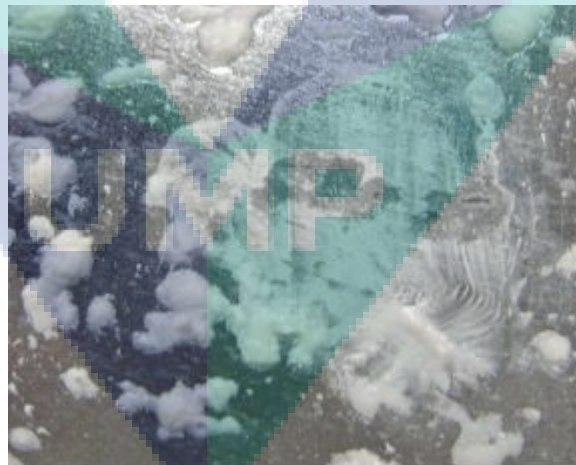
Figure 2.3-4: White rust on galvanized steel
