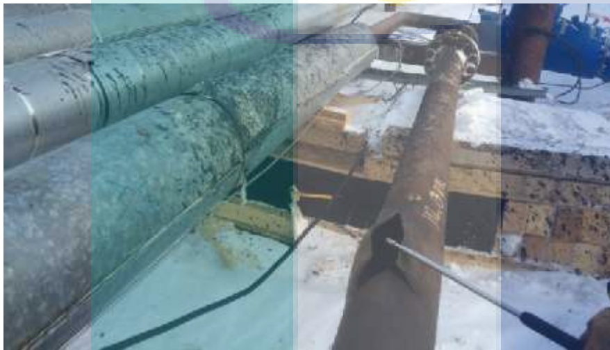
Figure 1.2: Example of a pipeline rupture.
