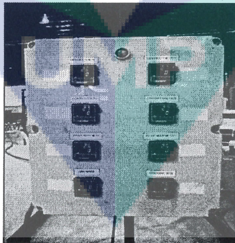
Figure 4.7: Temperature indicator of absorption chiller unit
