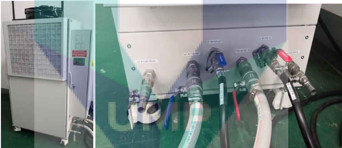
Fig 4-4. Chiller Set with Water Inlet and Outlet
