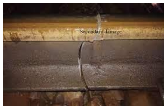
Figure 9. Horizontal cracking in the web. [38]
