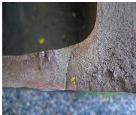
Figure 10. Longitudinal vertical cracking of the rail bottom. [42]
