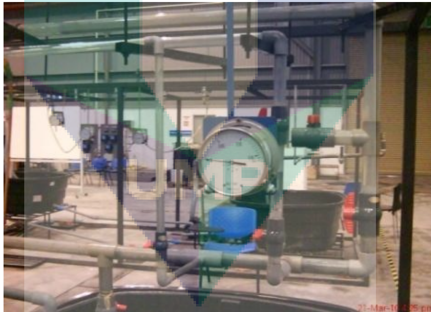
Figure 3.9: The differential pressure manometer.
