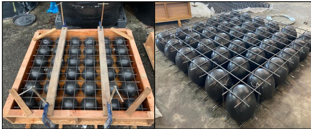
(a) Placing timber plank on top of the formwork (b) Iron wire tied between the top and bottom reinforcement lattice.
