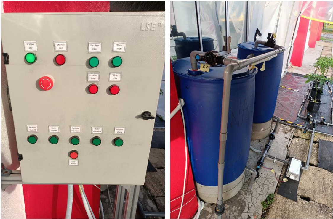
Figure 3.37 Figure for control panel and water tank
