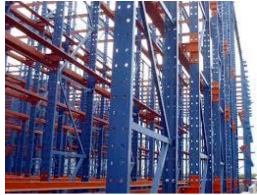
(b) Rack system
