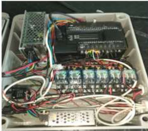
Figure 5: PLC and electronic components
