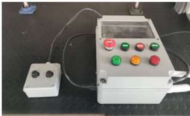
Figure 6: Joystick and PLC control box
