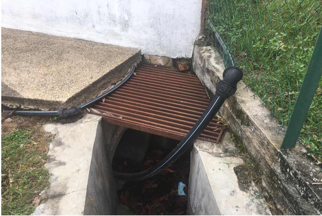
Figure 3.4(c): Discharge Outlet of UMP Gambang Mosque
