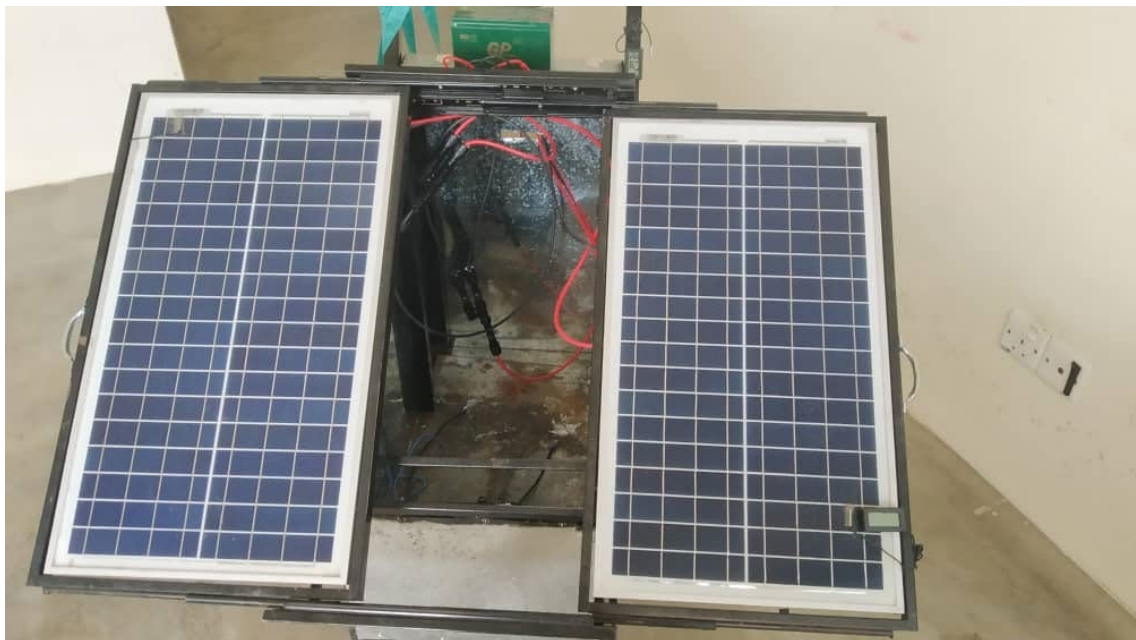
Figure 4.6 The real parallel connection of solar panels to solar charge controller.
