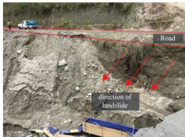
Fig. (1). The Bireuen-Takengon cross-road segment's experience of a landslide disaster, resulting in the collapse of a major section of the road.
