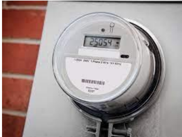
Figure 2.1 The Digital Meter Unit
