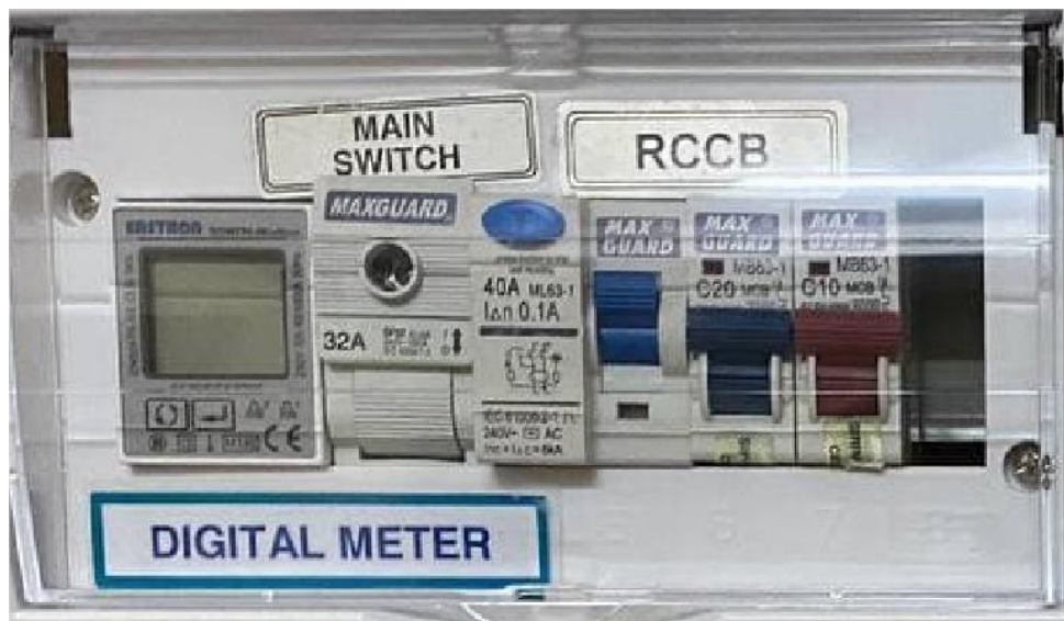
Figure 4.5 DB Box used in demonstration
