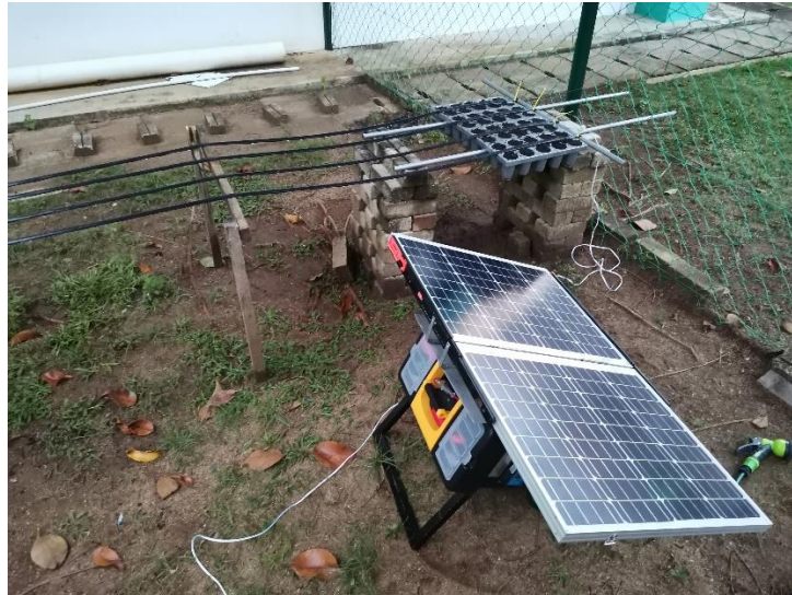
Figure 4.7 Solar Water Pump
