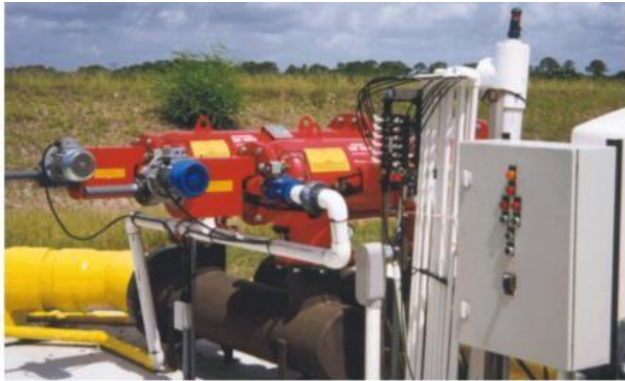
Figure 2.5 Control panel for automatically backflushing filters based on pressure differential between inlet and outlet of filter.
