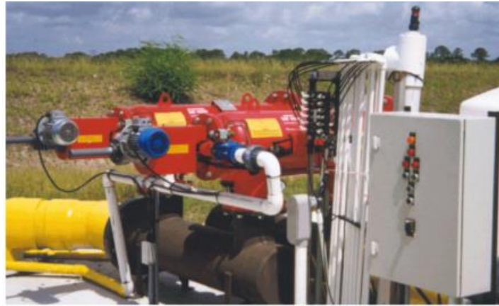
Figure 2.5 Control panel for automatically backflushing filters based on pressure differential between inlet and outlet of filter.
