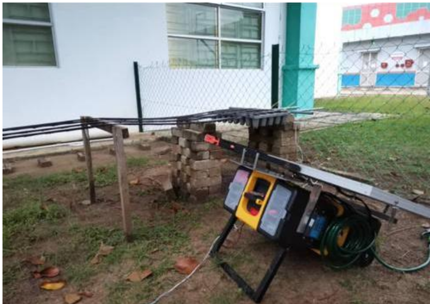
Figure 4.3 Setup at site
