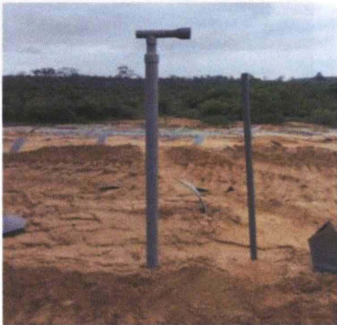
Figure 16 Installation of the stand of SSWT
