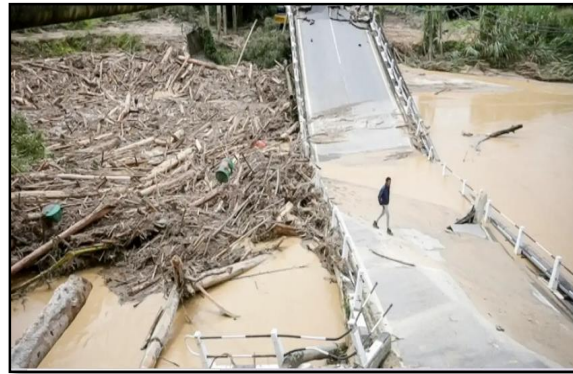
Figure 3. Slim River's bridge collapsed due to water surge at Slim River, Perak.
