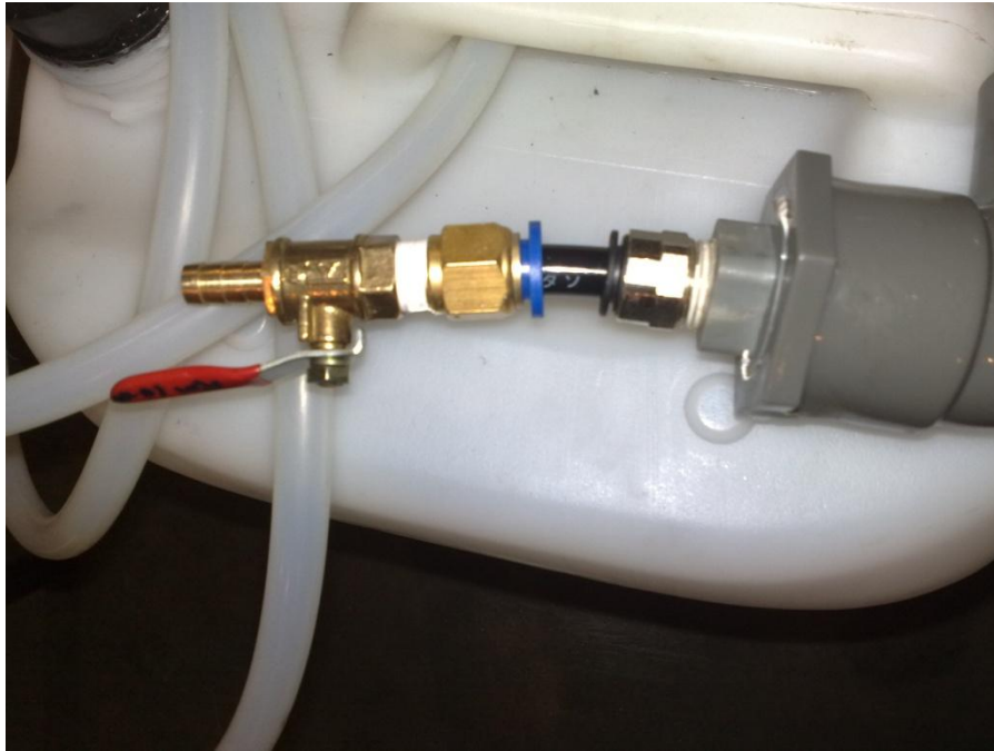
Figure 3.4: Connection between elbow and valve
