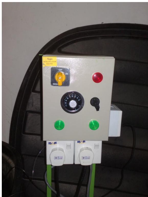
Figure 3.5: Temperature Control Panel Box
