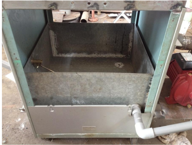
Figure 3.23: Water tank for cooling tower
