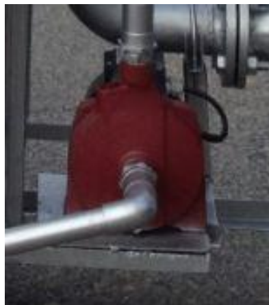
Figure 3.12: Circulating pump for cooling tower
