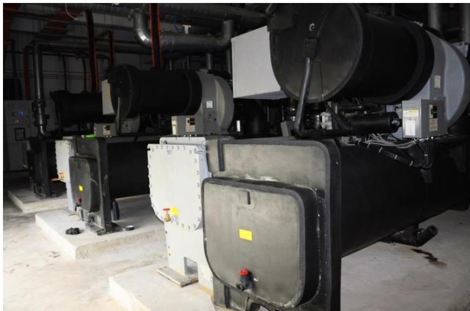
Figure 2.8: Centrifugal chiller in FKM building
