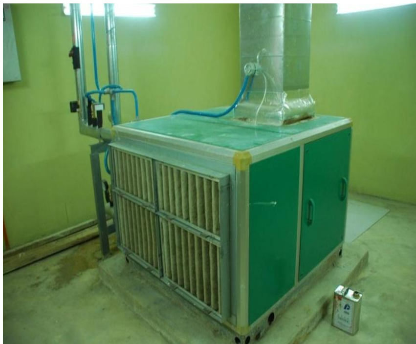
Figure 2.9: Air Handling Unit in FKM building
