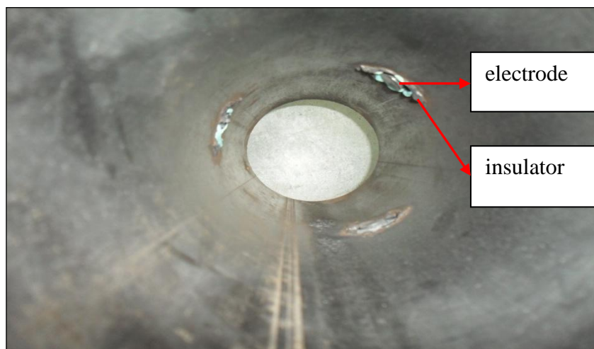
Figure 3.4: Implemented of electrode in pipeline
