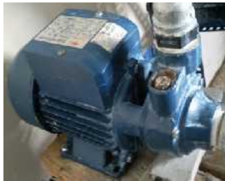
Figure 3.5: Circulating Pump with Electric Motor
