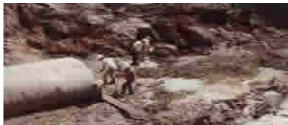
Figure 2.14: Sanitary Sewer Pipelines
