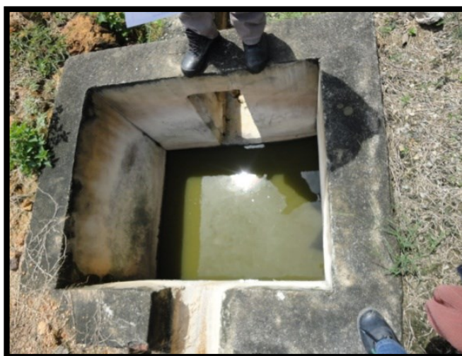
Figure 3.3: final effluent discharge at ponding system
