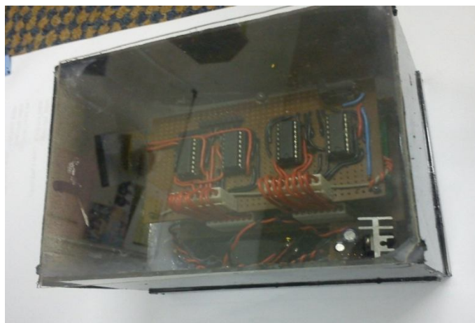
Figure 3.13 : Main circuit box
