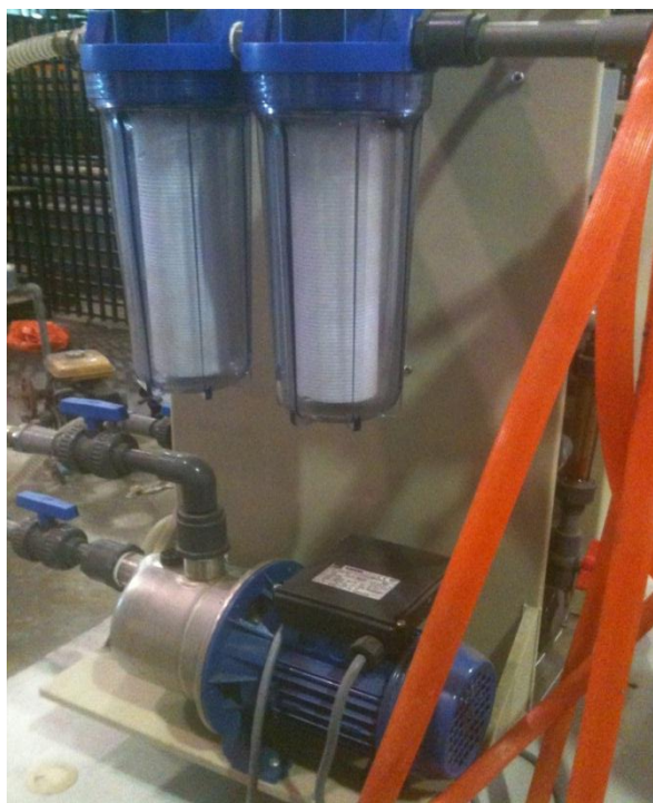
Figure 3.4: Electrocoagulation OT-1 installed with pump and filter
