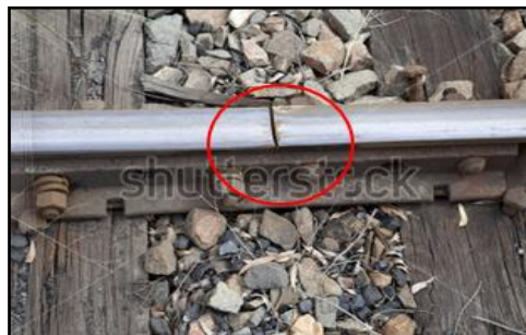
Figure 1.4: Crack on railroad
