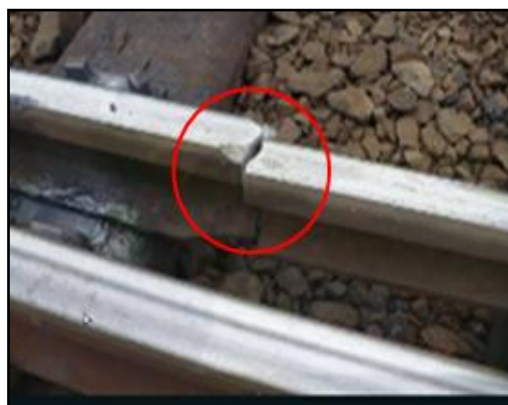
Figure 1.6: Serious crack on railroad
