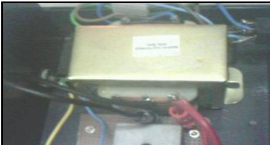
Figure 4.5 : Transformer 3Amp, 56Volt
