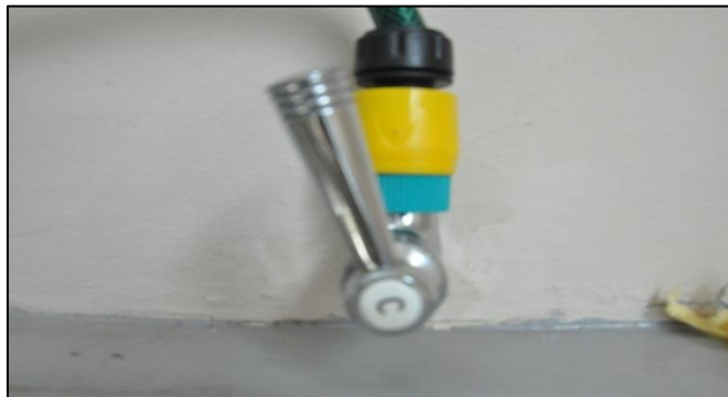
Figure 3.38: Pipe is opened at 15^\circ
