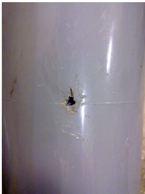
Figure 4.3 Cracked defected tee
