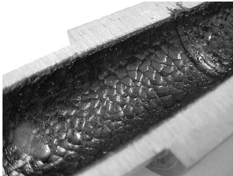
Figure 2.3 Degradation of CPVC pipe caused by prolonged exposure to hot concentrated sulphuric acid
