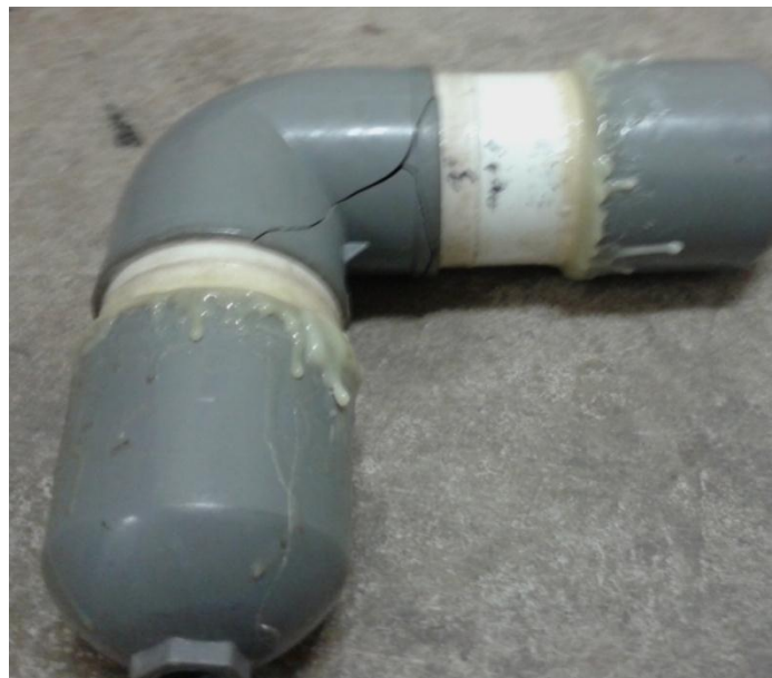
Figure 4.1 Cracked perfect elbow
