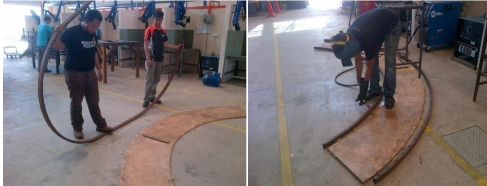
Figure 3.6: Steps to build the mold for the reinforcement on the curved tank.
