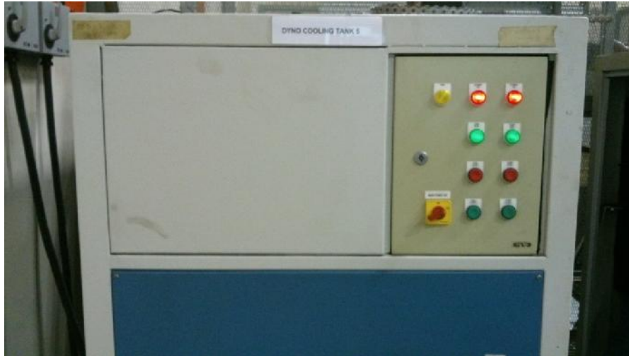
Figure 3.17: Cooling tank for Dynamometer
