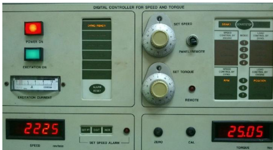
Figure 3.22: Torque reading on the main control panel
