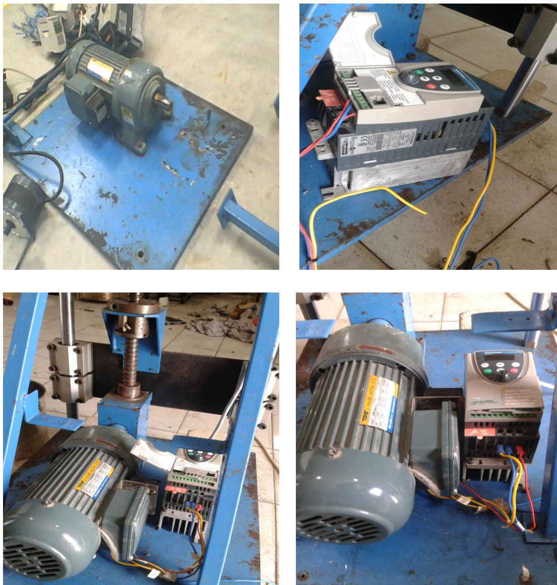
Figure 4.40 3 phase motor and inverter
