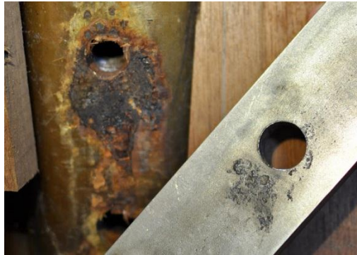
Figure 2.2: the pitting corrosion on the back of the pipe and in the background.
