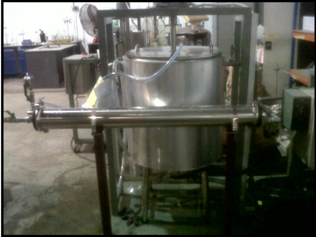
Figure 3-4: Reverse osmosis membrane system
