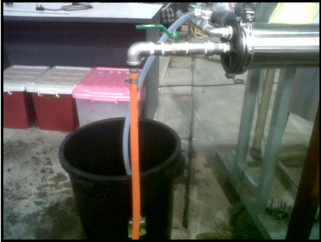
Figure 3-8: Membrane was cleaning using backwashing method
