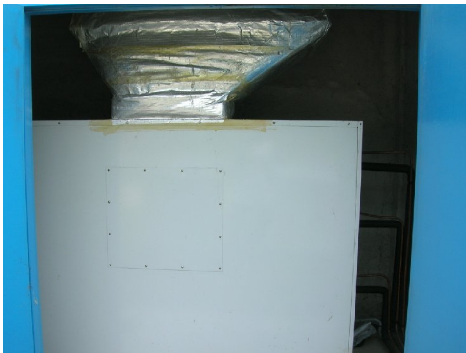
Figure 4.8: Package unit at WDKU
