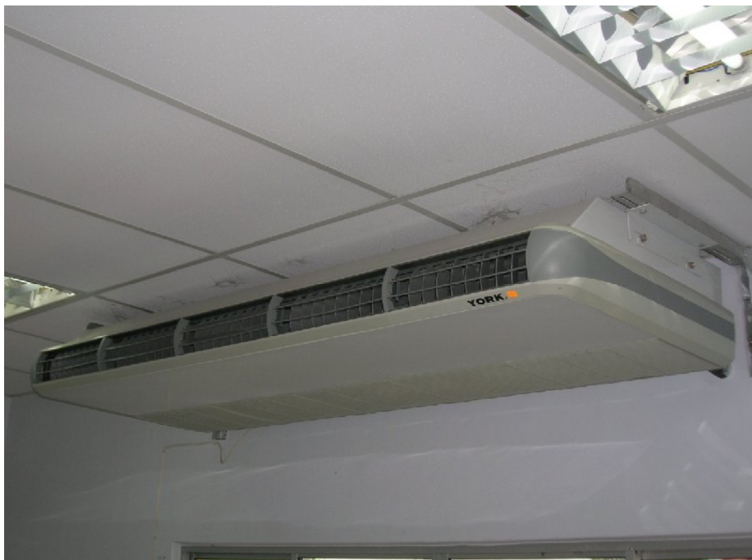
Figure 4.7: Split unit at WDK
