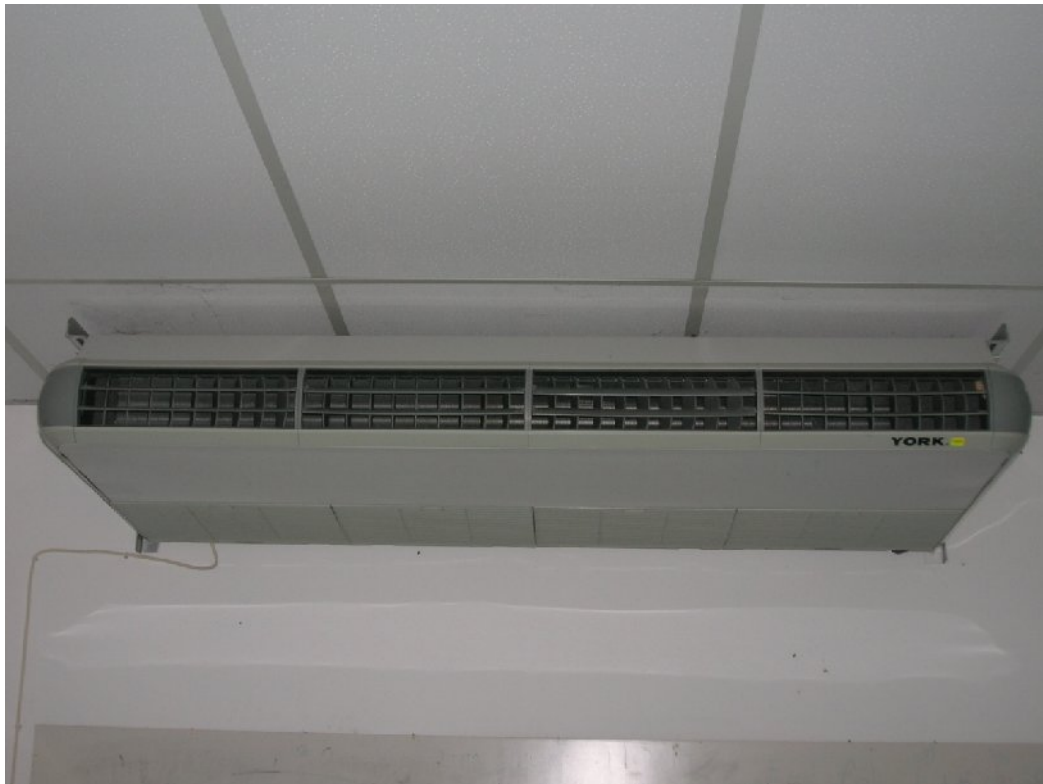
Figure 4.6: Split unit at WBK
