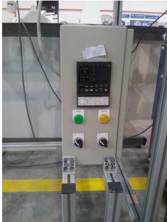
Figure 3-5: Control system of Pyrolyzer used
